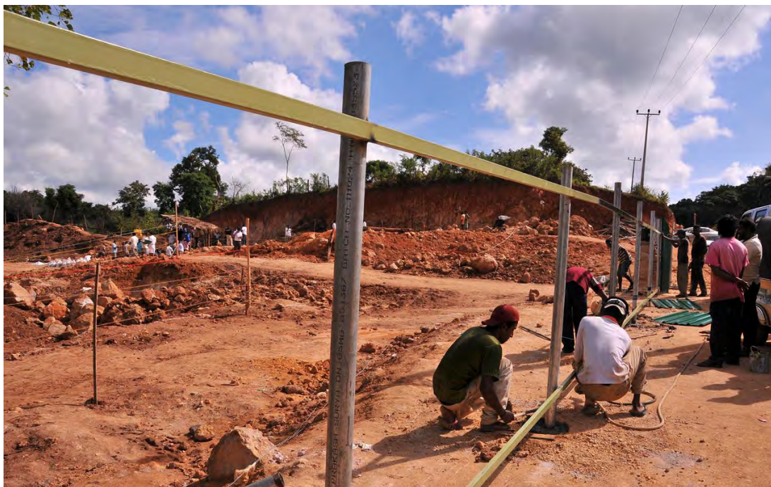
Figure 16: On March 1, 2012, the mining site is prepared by the NGJA. Photo: Andrea Heather Go.
