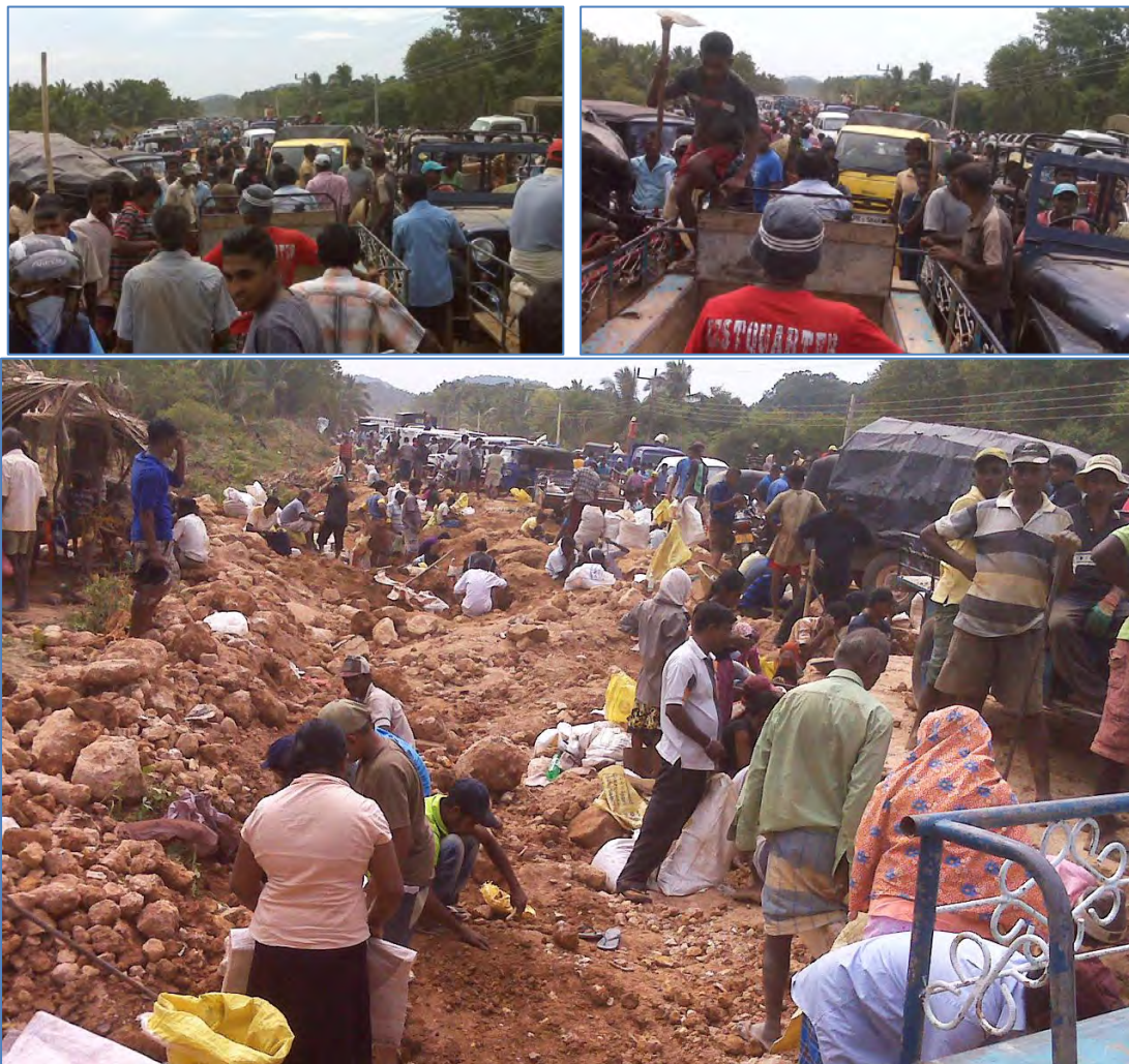
Figure 8: Local people rushed to the road construction site near Kataragama on Feb 14, 2012. A frenzied mining effort using hand tools or even bare hands soon commenced. Photos: Eranga Basnayake.
