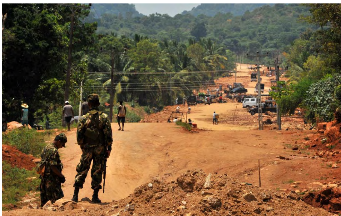
Figure 11: The road construction site where the discovery was first made, as seen on March 8, 2012. Photo: V.Pardieu / GIA Laboratory Bangkok.
